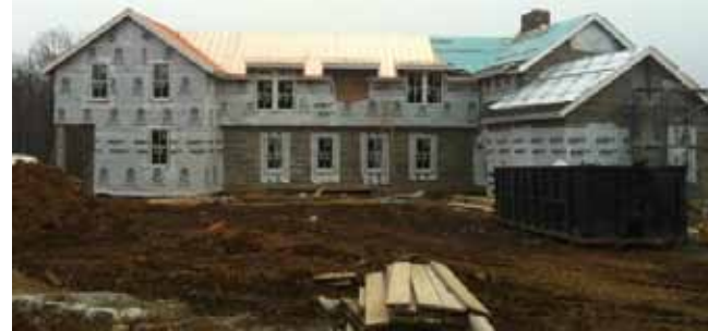
Work underway on the Headmaster's House on the Martinsville Campus. Courtesy of Pingry Communications
